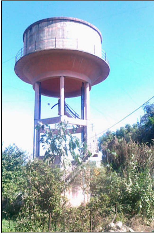
Fig 3: An Overhead Water Supply Tank in Dewas town, the new water augmentation project for the town, looks to add a few more of these to increase the storage capacity.
